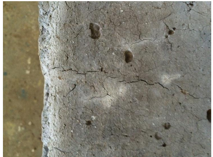
Figure (4): Typical of Fire Cracks Distributed Randomly over The Specimen
