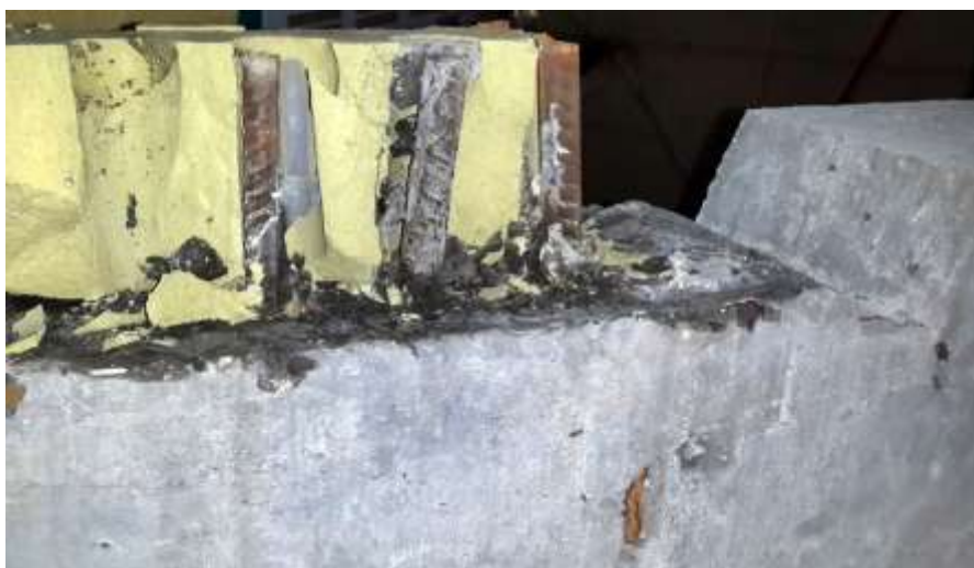
Photo (3): Failure of concrete to Bricks with six dowels
